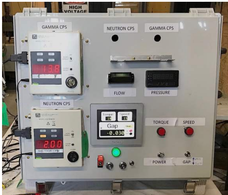
Sample of a Remote Control Station
